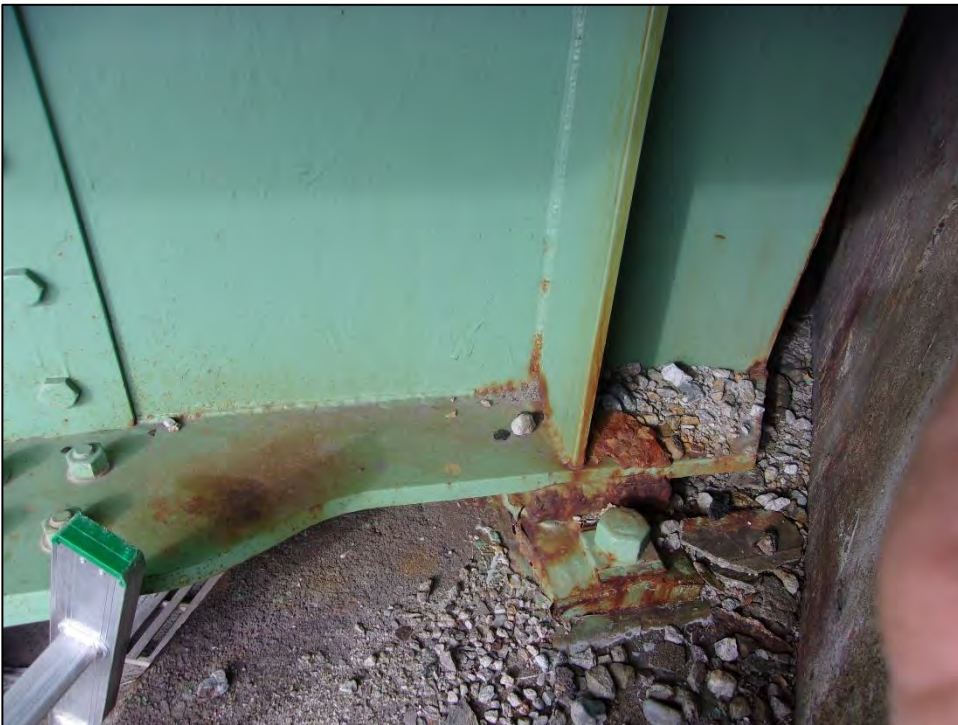
Photo 6: View of the south face of girder "G" at the east abutment of Bridge No. 904. There are narrow gaps between the face of the backwall and the backside of the steel girders that could provide potential roosting areas. Photo date: November 2017
