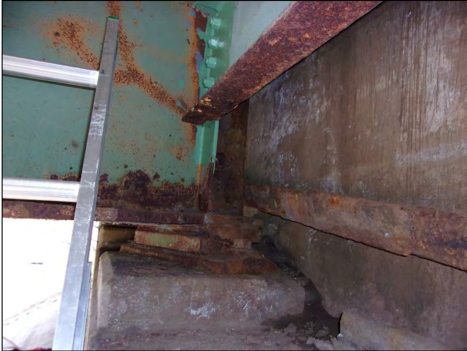
Photo 3: A view of the steel girder and bearing at the east abutment. The crevices in this section of the bridge may provide limited roosting opportunities for bats.
