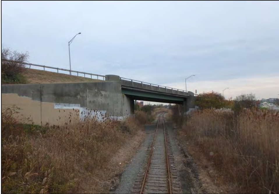
Photo 7: A view of Bridge No. 905 looking north. Bridge No. 905 is a one-lane bridge conveying the Route 138 westbound on-ramp to the Pell Bridge over Newport and Narragansett Bay Railroad ROW. This bridge is scheduled to be removed.
