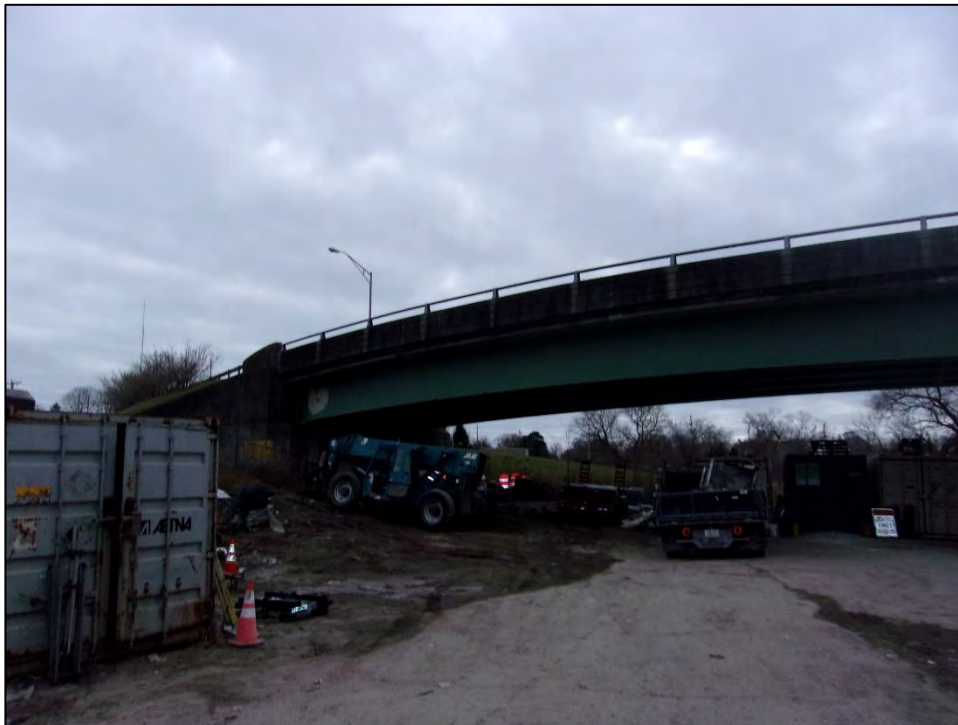
Photo 10: A view of Bridge No. 906 looking south. Bridge No. 906 is a one-lane bridge that conveys Route 138 eastbound to the Downtown off-ramp that connects to J.T. Connell Highway. The bridge spans the Newport and Narragansett Bay Railroad ROW and an abandoned ramp. This bridge is scheduled to be removed.
