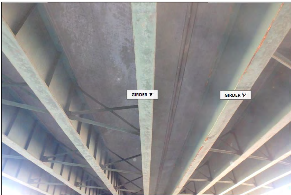
Photo 16: A view of the underside of Bridge No. 906. This bridge has a reinforced concrete deck supported by steel girders. Photo date: November 2016
