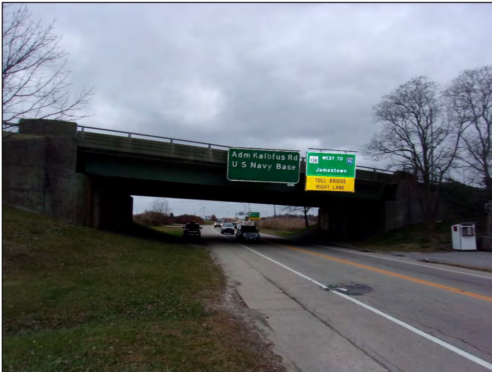
Photo 12: A view of Bridge No. 907 looking northerly. Bridge No. 907 is a two-lane bridge conveying Route 138 off/on ramp over J.T. Connell Highway and it is scheduled to be rehabilitated. Photo date: November 2017
