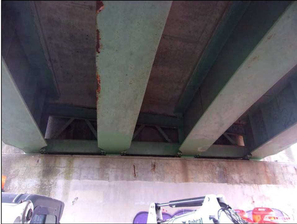
Photo 11: A view of the underside of Bridge No. 906 looking towards the east abutment. The bridge has a reinforced concrete deck supported by four steel girders. The underside provides limited suitable roosting space. Photo date: November 2017
