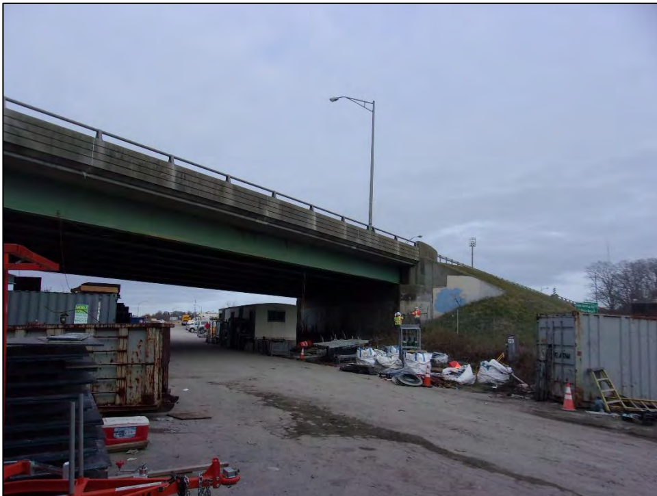
Photo 4: A view of Bridge No. 904 looking northeasterly from the abandoned ramp. Bridge No. 904 is a two-lane bridge that conveys Route 138 off/on ramp over Newport and Narragansett Bay Railroad ROW and an abandoned ramp. This bridge is scheduled to be rehabilitated.
