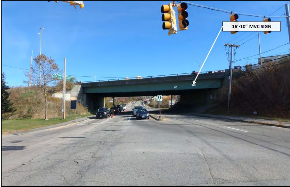
Photo 15: A view of Bridge No. 908 looking south. Bridge No. 908 is a two-lane bridge conveying Route 138/238 over Admiral Kalbfus Road. This bridge is scheduled to be removed. Photo date: November 2016
