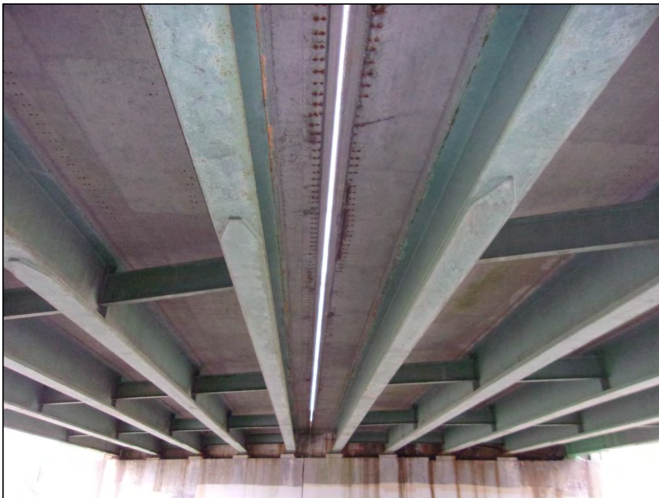
Photo 2: A view of the underside of Bridge No. 903. The bridge deck is concrete supported by steel girders. Photo date: November 2017
