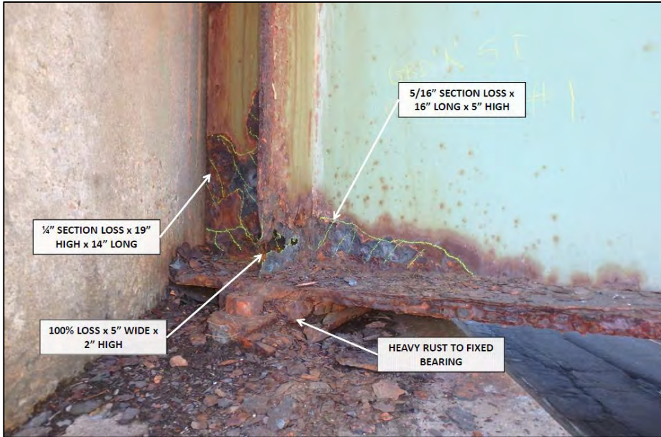
Photo 17: A view of one of the girder ends at the west abutment. There are narrow gaps between the backside of the girder and the face of the backwall and between the bottom of the girder and the top of the bridge seat that may provide potential roosting spaces for bats.
