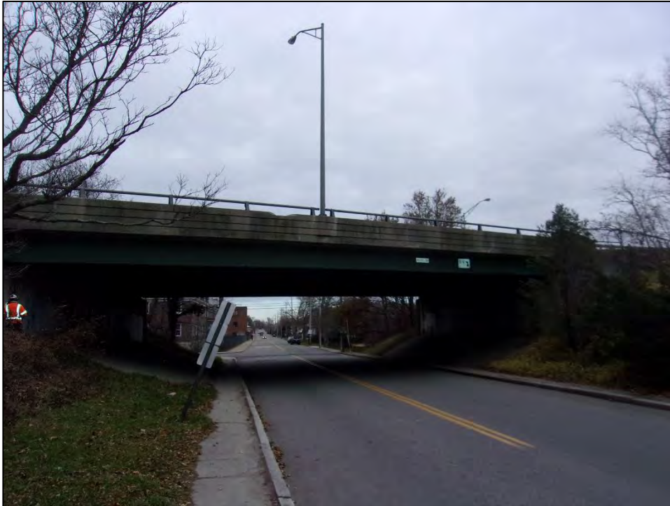
Photo 1: A view of Bridge No. 903 looking south. Bridge No. 903 is a four-lane bridge conveying Route 138 off/on ramp over Third Street. This bridge is scheduled to be rehabilitated. Photo date: November 2017
