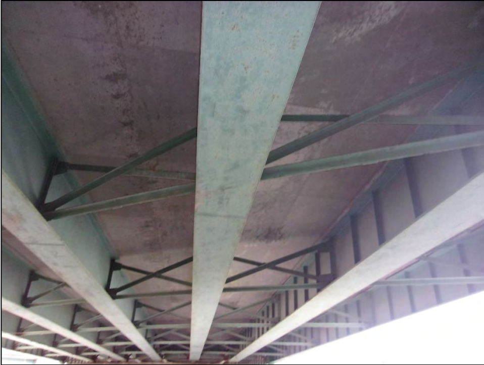
Photo 5: A view of the underside of Bridge No. 904. The bridge has a reinforced concrete deck supported by seven steel girders. The underside provides limited suitable roosting space. Photo date: November 2017
